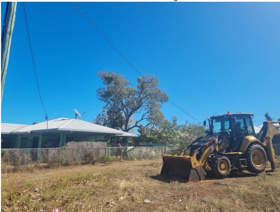
Photo 2 – Overhead cable preventing excavation of TP2
