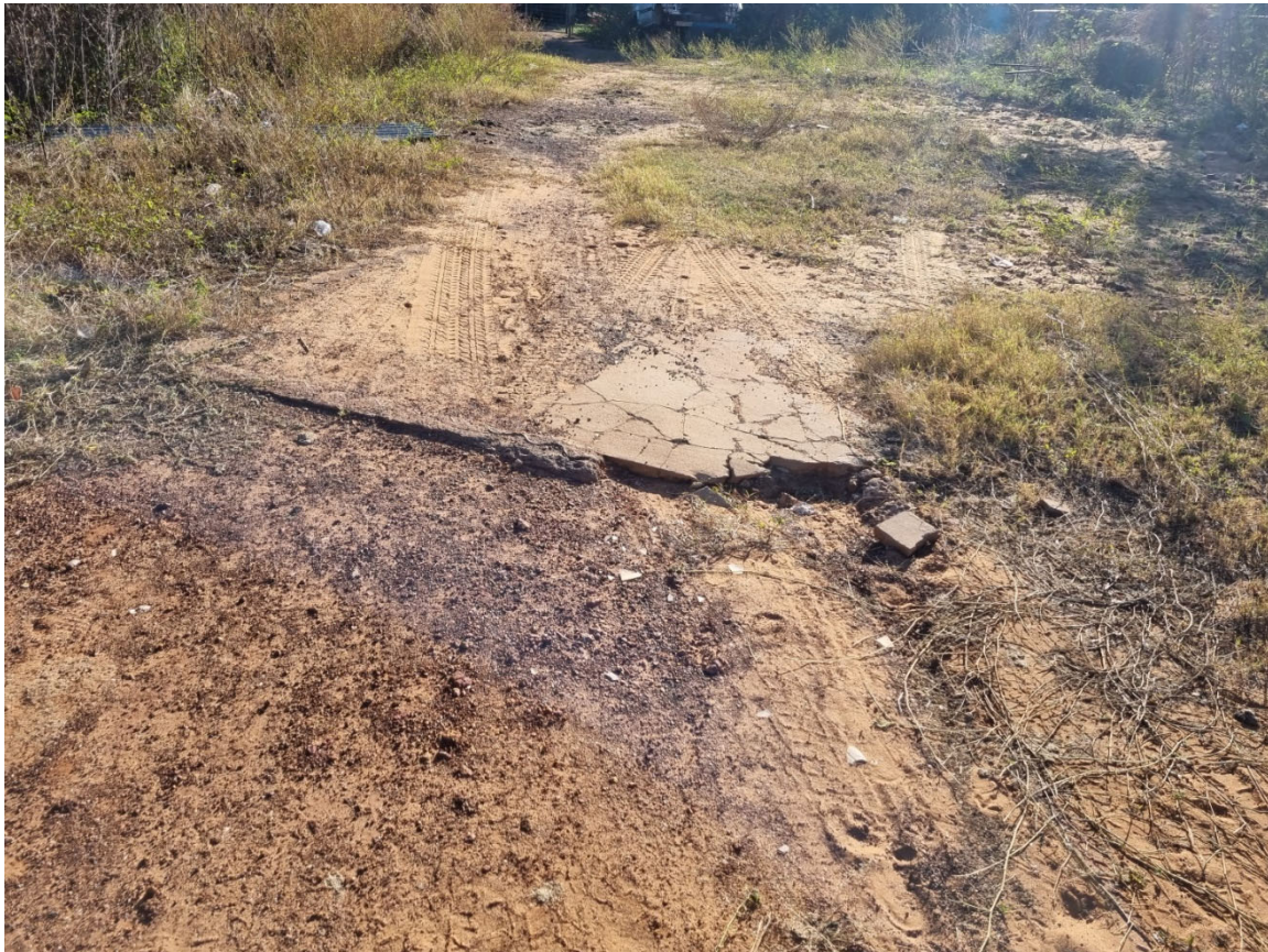
Photo 3 – Exposed concrete slab
