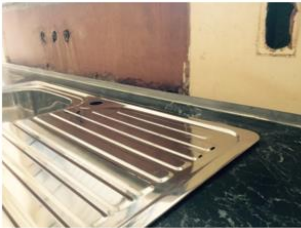
Benchtop is placed in position. Stainless steel plate is to be the length of the bench top or a minimum 2.4m long and be a minimum of 1.2m from each side of centre of new sink
