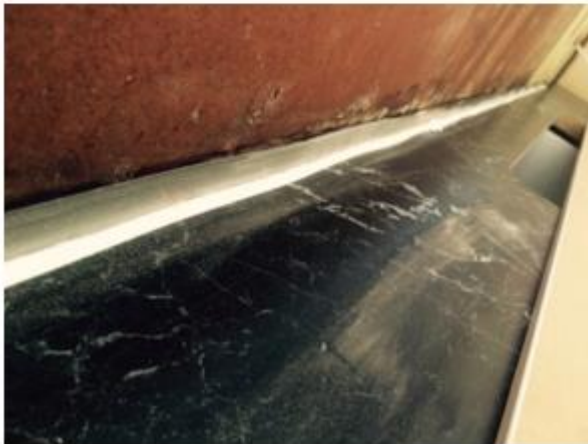
A bead of "Sikaflex" is applied to join of the stainless-steel plate and the bench top, then the splashback is put in position
